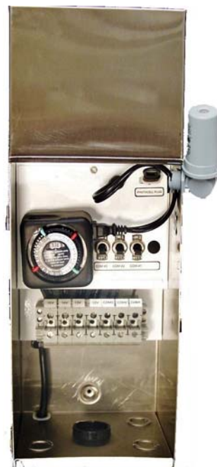
Figure 3 – 24 hour clock timer and photocell installation
